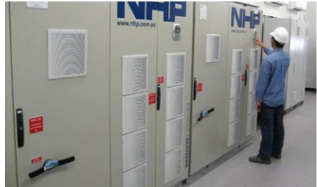
(above) Clean louvers allow optimum air flow
