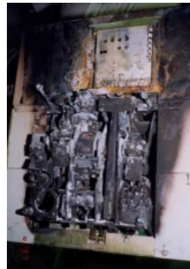
(above) Damaged switchboard from the Goliath
