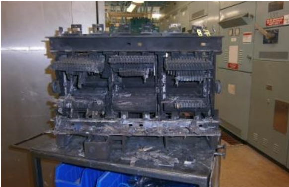
Figure 4 – Fire damaged ACB caused by an overheating cluster
